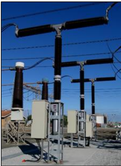
Circuit breakers in an electrical substation.
